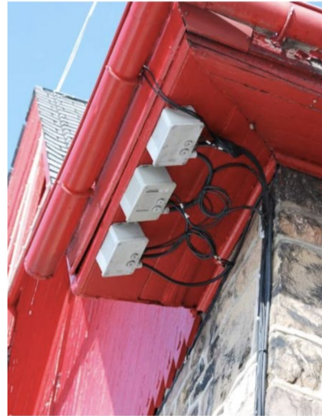
Cables exit power supply from top.
