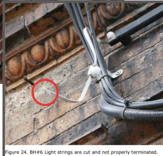
Figure 24. BH#6 Light strings are cut and not properly terminated.
