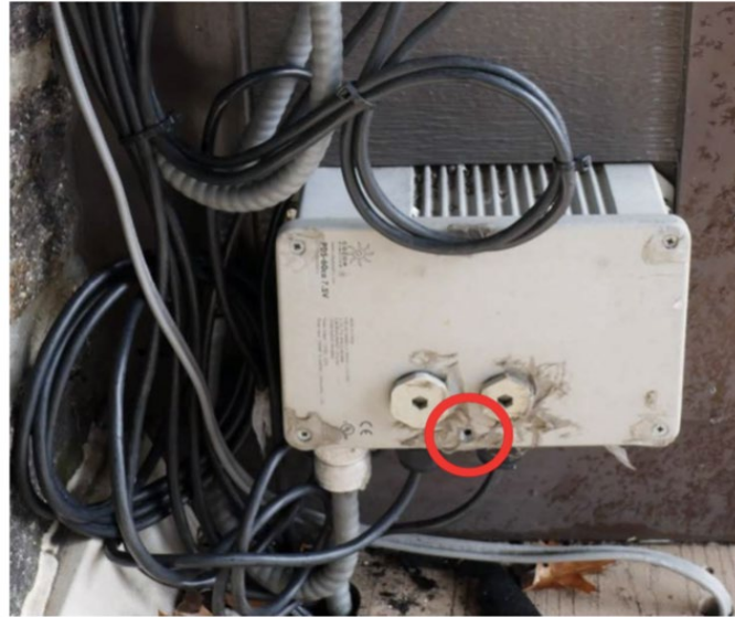
Figure 16. BH#4 Power supply cover plate missing screws.
