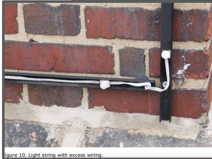
Figure 10. Light string with excess wiring.
