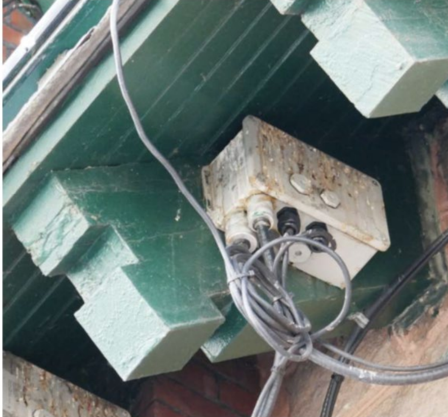
Figure 46. BH #13 Power supply with bird feces.
